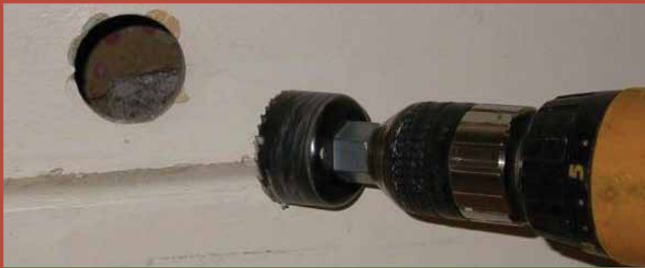
A drill can be used to take a core sample for lead testing.
