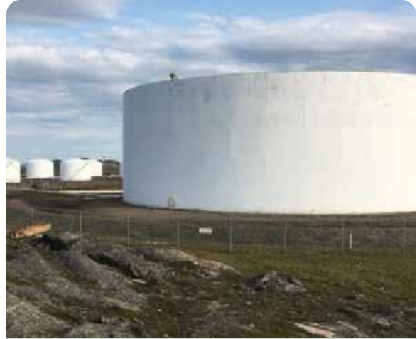
Lead paint was often used on industrial structures like tank farms
