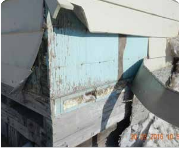
Lead paint can be found on old buildings
