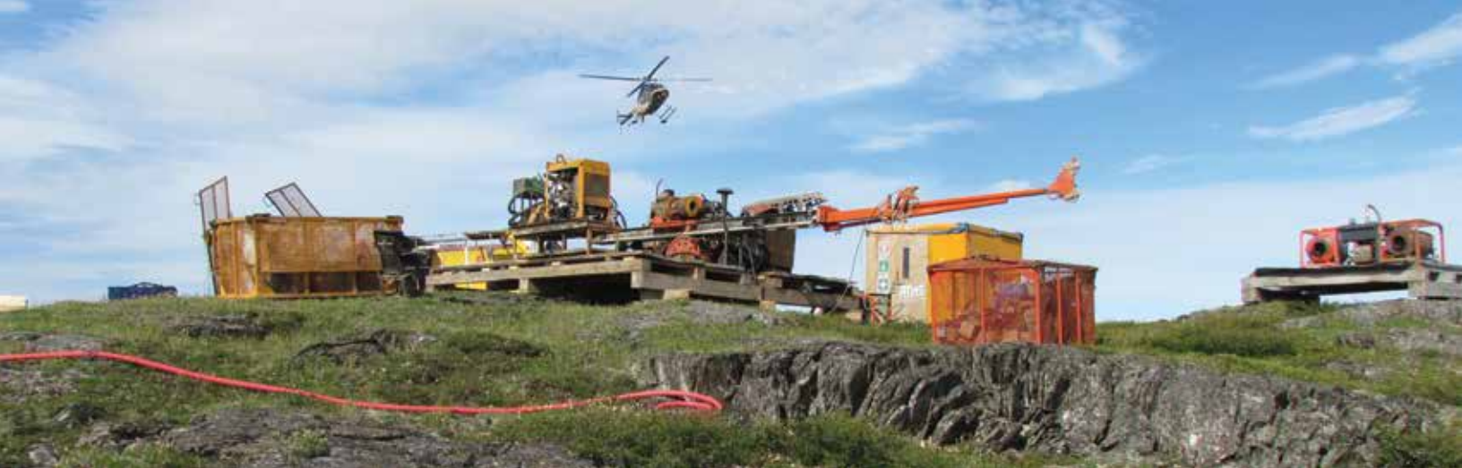
Constructing the first drill pad of the season at Western Atlas' Meadowbank gold project. Courtesy of Western Atlas Resources Inc.
