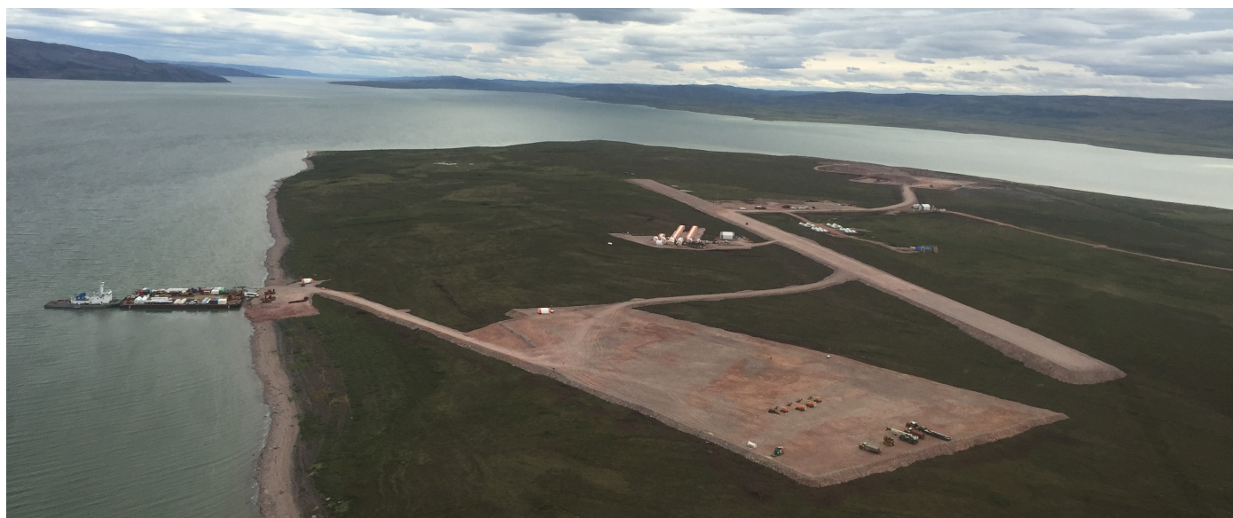
Barges unloading at the Marine Laydown Area, Back River project. Courtesy of Sabina Gold and Silver Corp
