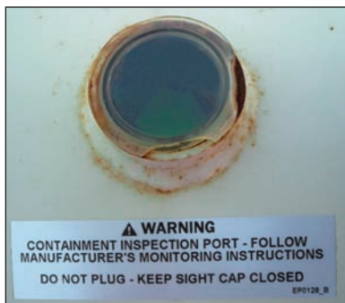
5.2c Inspection port on a double-bottom tank. Note the green coloured indicator – this indicator will turn red if the inside bottom leaks.
