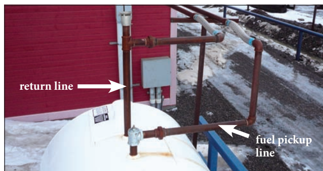
6.3a Commercial double-wall steel heating oil tank showing the pickup and return fuel lines.
