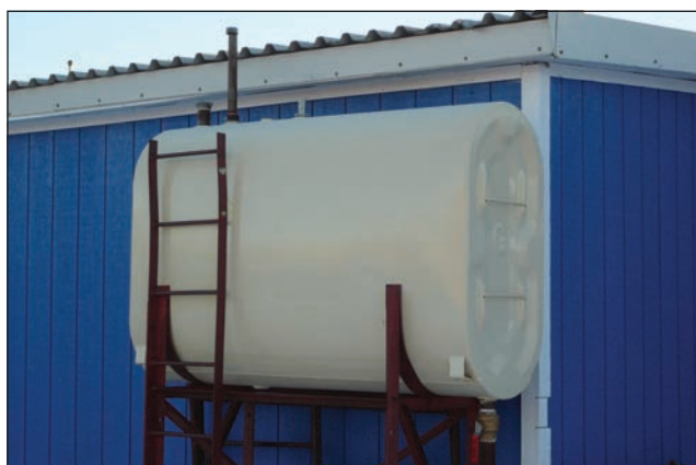
5.2 Single wall, double bottom steel heating oil tank.
