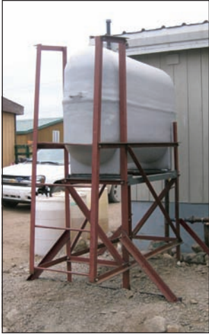
4.5c Note the tank stand modification: the owner has broadened the base of the metal tank stand and added reinforcing struts at 45 degree angles to further strengthen the base. This has provided significantly more stability to the installation than would be afforded by the original unmodified stand.
