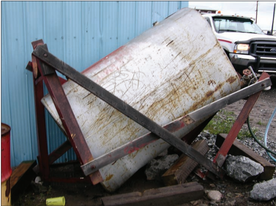
4.5b This heating oil tank was resting on a wood-metal stand, which eventually collapsed under the weight of the tank, spilling 445 litres (100 gallons) of heating oil onto the ground.
