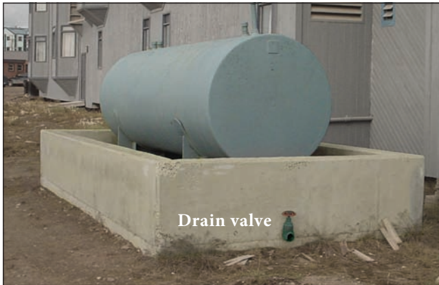
4.12 4,550 litre (1000 gallon) tank with a concrete berm. Note that the drain valve is not fitted with a lock or chain and thus can be tampered with.
