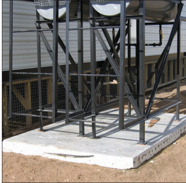
4.5d A twin tank installation firmly secured to a full concrete pad. This provides a solid foundation.
