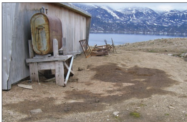
4.10 Excessive ground staining from a poorly installed and maintained oil tank.
