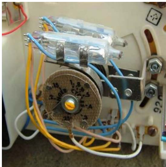
Figure 11 – Interrupteurs à mercure Source : California Department of Toxic Substances Control
