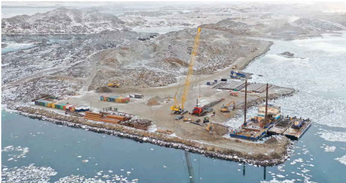
Progress on the new Deep Sea Dock and lay down area at Iqaluit
